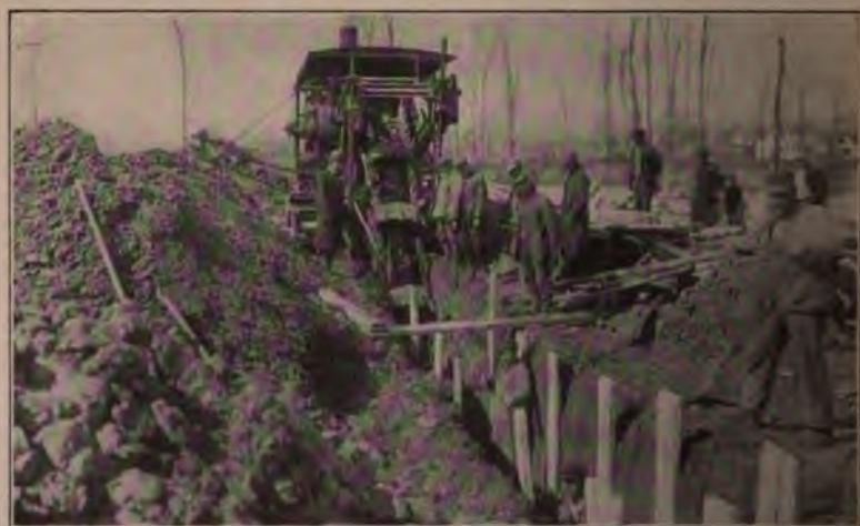
Chicago (Austin) Trench Excavator Digging a Trench 26 inches wide and 15 feet deep. Figure 119.
